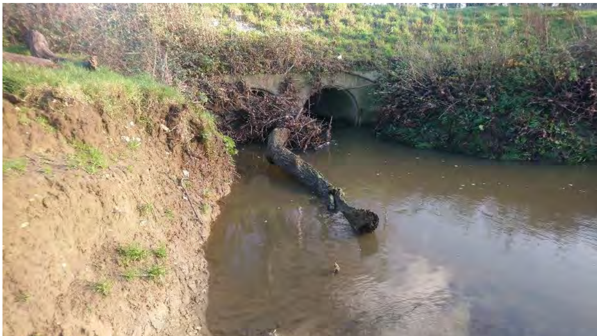
Photo 4. The inlet of a partially blocked culvert bridge, subsequently cleared out by the volunteers.
